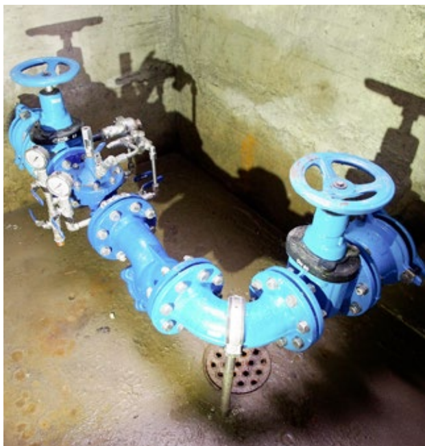
Neue DRV-Station GLA – VAL DN80
