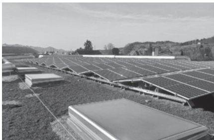
Photovoltaikanlage Turnhalle Haslen
